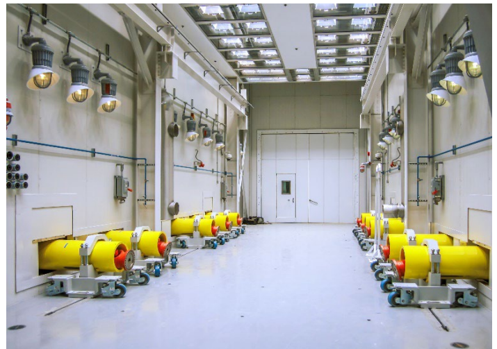
PEVEL - Test Cell Interior
